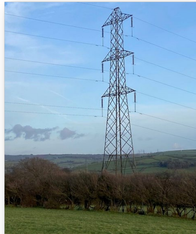
Onsite pylon in Solar Area East, providing the point of connection
