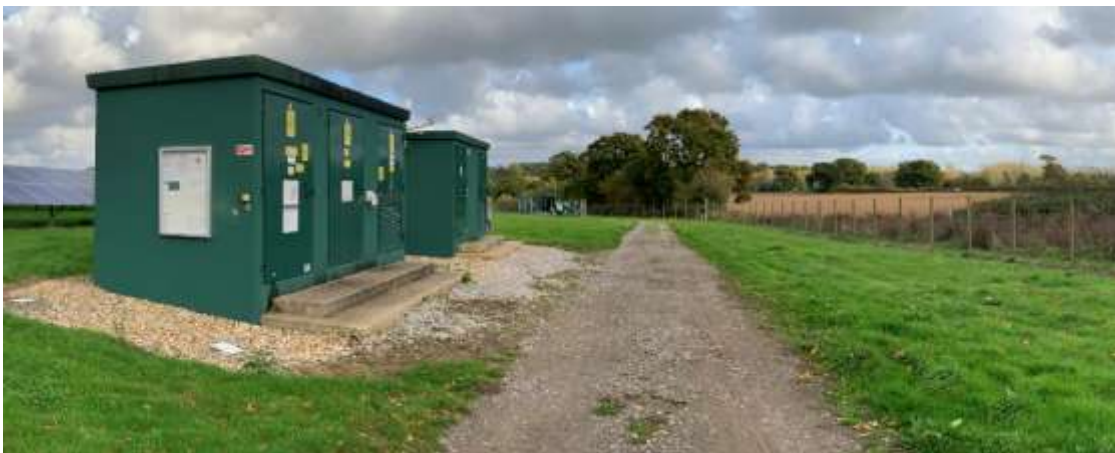
Insert 32: Typical Transformer
