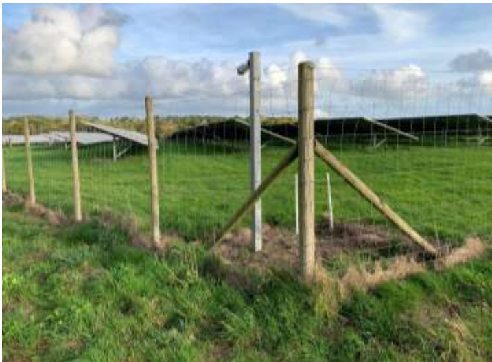
Insert 44 and 45: CCTV Poles and Fencing
