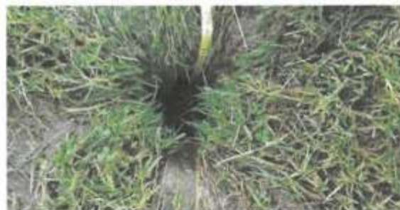
Figure 17. A 'blow hole'
