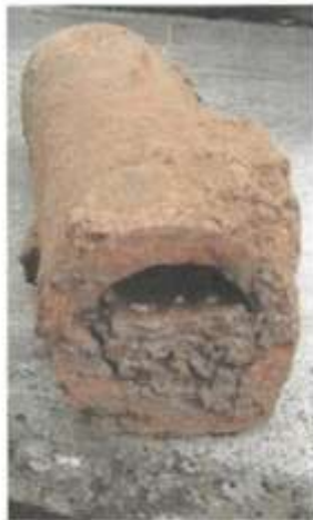
Figure 22. Silted clay drain
